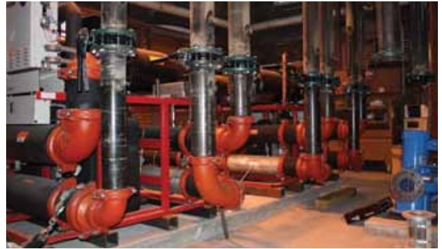
Building 336 main mechanical room
